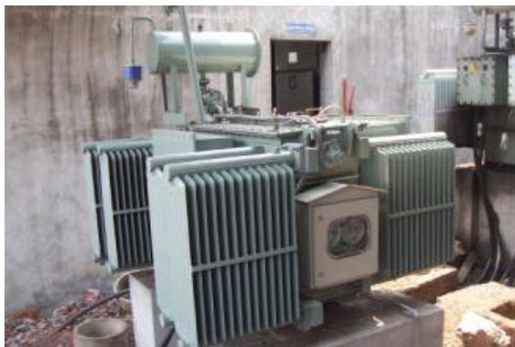
Energy efficient transformer
