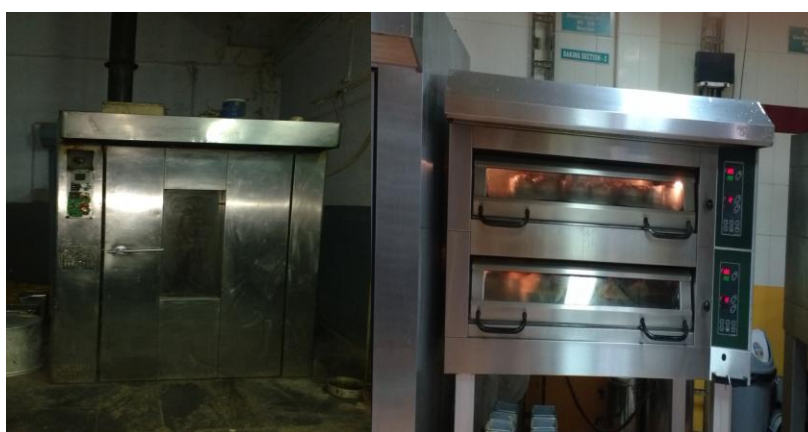
Diesel fired oven
